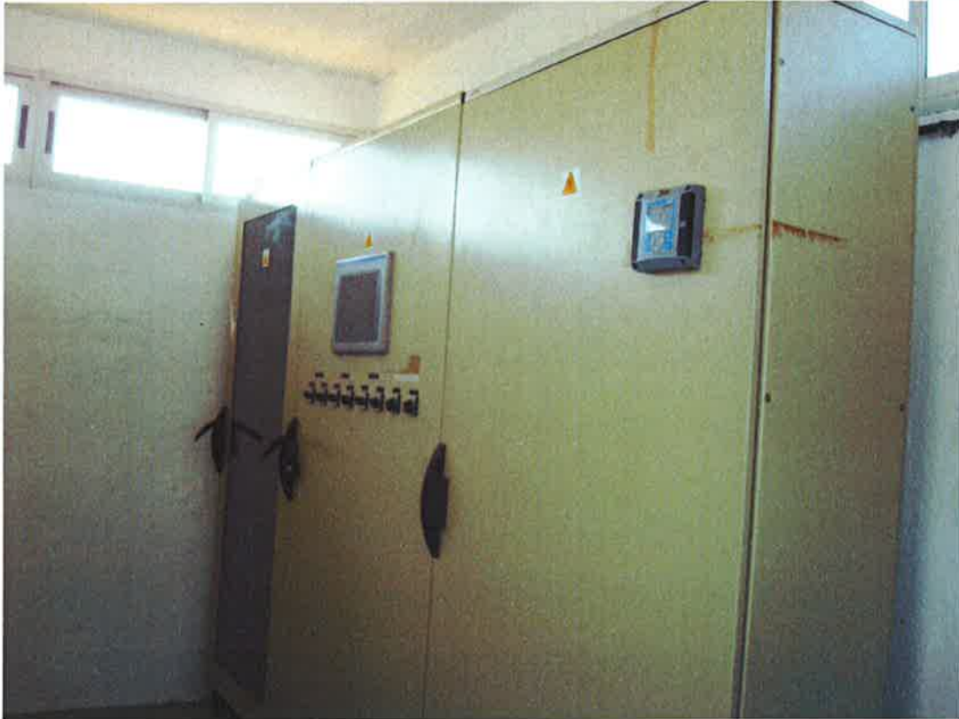
Vista frontal del PLC-1LL.
