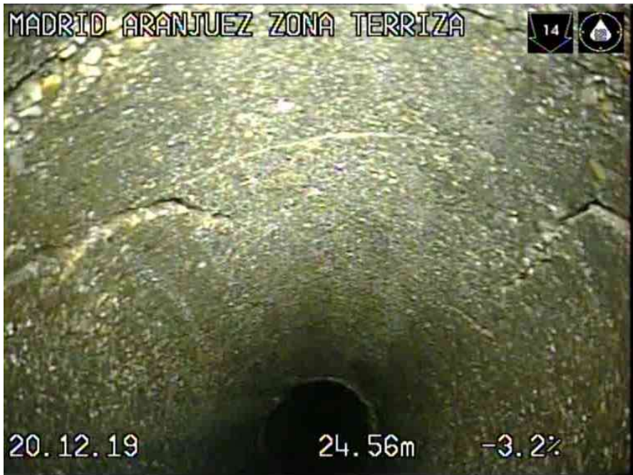
MADRID ARANJUEZ ZONA TERRIZA 1_c15a27c9-3181-408b-be8f-c5bc363e7892_20191220_121717_192.jpg, 00:02:15, 24.56 FISURA PUNTUAL
