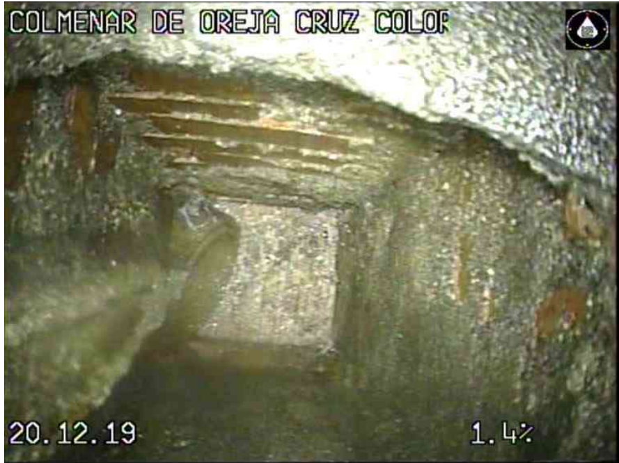
3_e5afe212-86b4-4a32-b587-d5a6d3d1210a_20191220_092109_781.jpg, 00:01:11, 8.20 ACOMETIDA EN TECHO SOBRESALIENTE a 12
