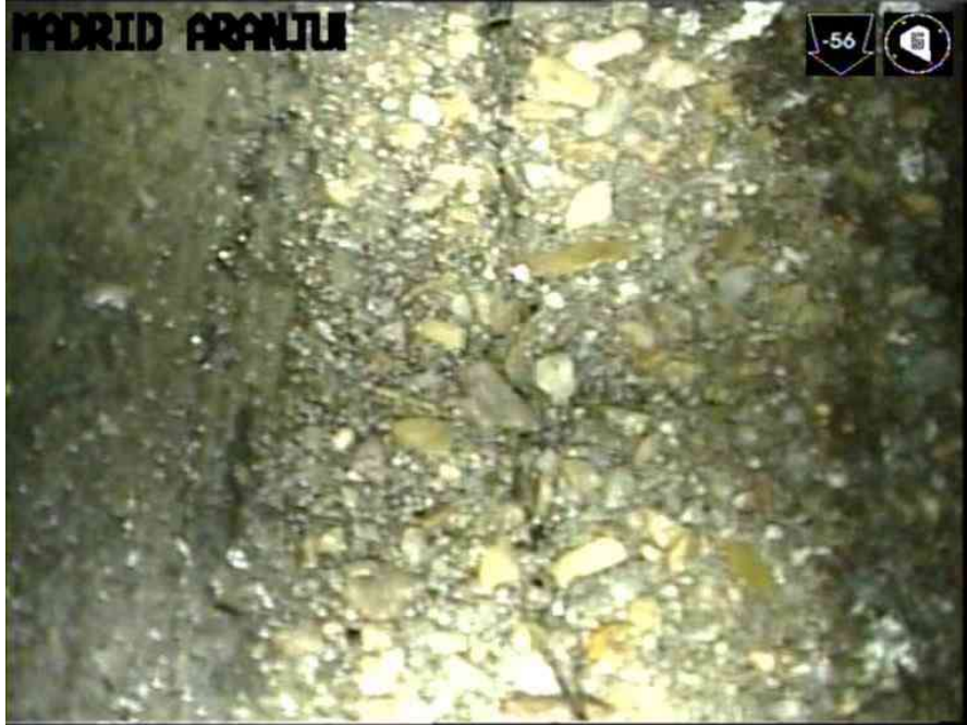
2_ cefeb85d-fbd1-4957-82cb-603a503ca965_20191220_124150_959.jpg, 00:02:17, 25.91 FISURA PUNTUAL
