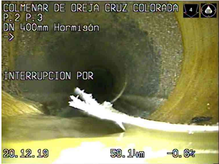
2_b59055ed-6017-40bf-8bab-5484b419477b_20191220_090343_127.jpg, 00:05:48, 59.14 REPARACION POR MANGA TOTAL MAL INSTALADA
