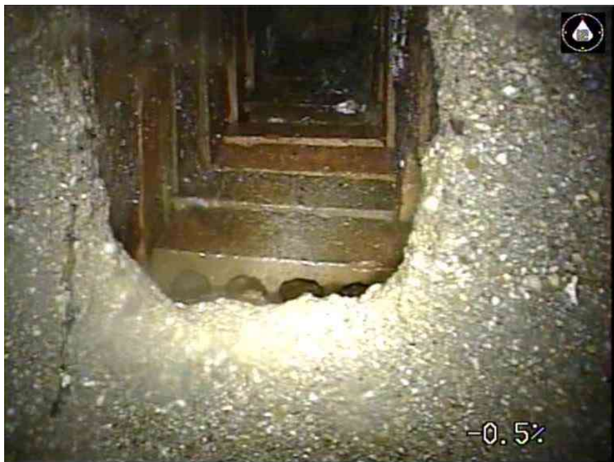
4_dd0721ba-15f9-463f-b018-d3168fb6bedb_20191220_092602_158.jpg, 00:02:14, 25.65 ACOMETIDA EN TECHO SOBRESALIENTE a 12
