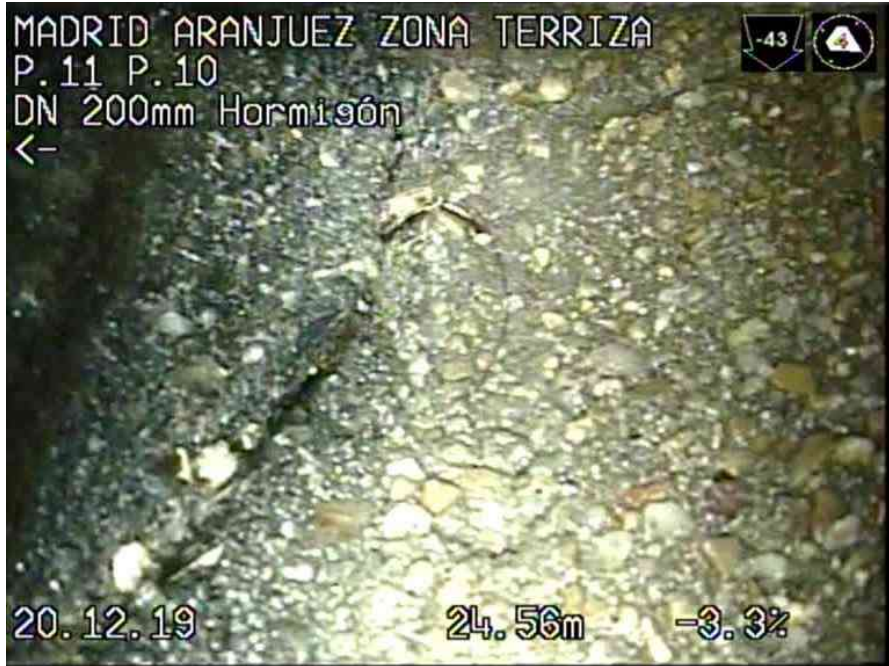
1_c62cbd21-7869-4072-9774-738c5ef32eab_20191220_121728_387.jpg, 00:02:15, 24.56 FISURA PUNTUAL
