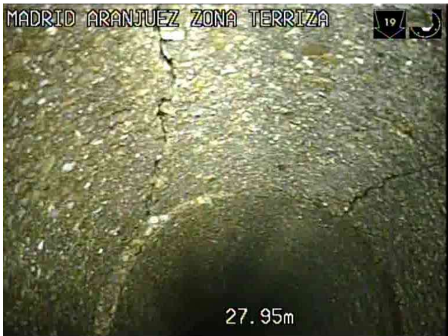
1_73fa466f-3692-465f-82b5-81593e8fa6ae_20191220_121803_639.jpg, 00:02:56, 27.95 FISURA PUNTUAL
