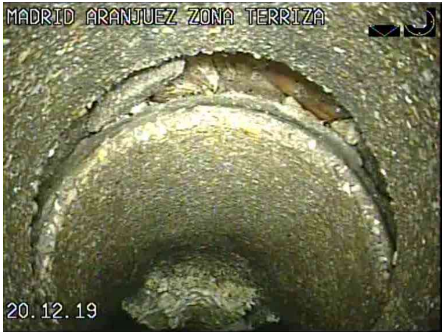
1_8db6046c-113c-4608-86ac-5c5e3a286b56_20191220_121957_145.jpg, 00:03:48, 32.73 TUBERÍA HUNDIDA
